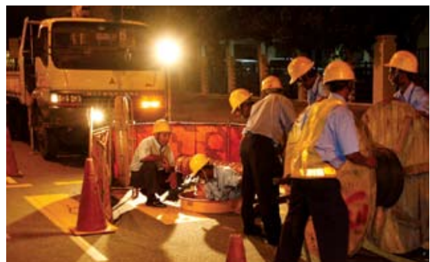
In 2008, Metro Ethernet covered 23 access rings and linked 110 buildings in Colombo.
