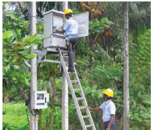
MSAN installation under the i-Sri Lanka programme
